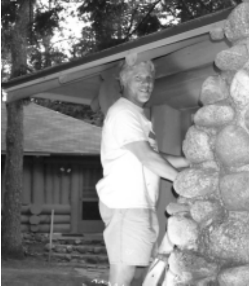
This summer Gary replaced the old chinking between the logs of the Dining Hall and Kitchen building.
